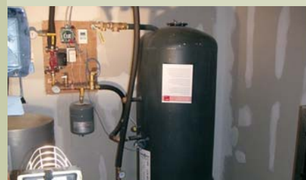
Super-insulated solar and hot water tanks.
