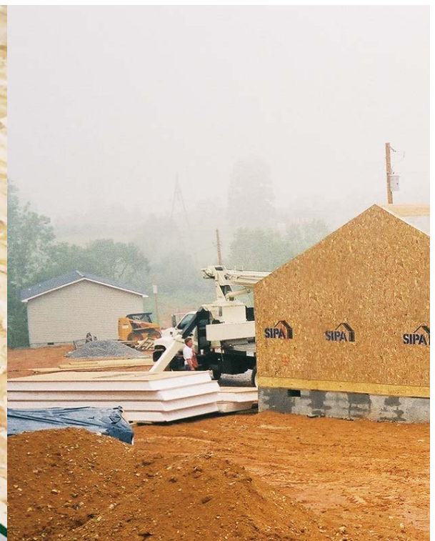
Habitat for Humanity volunteers prepare to place roof panels for a zero-energy home (ZEH). The spanning capabilities of SIPs allow a single ridge beam to support the roof, meaning less joints and an overall airtight structure.
