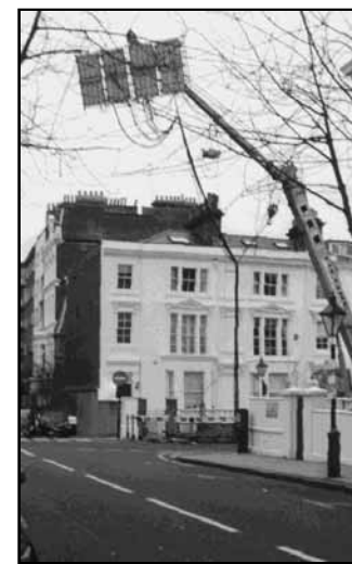
The big crane with the strong floodlights was positioned in Vicarage Gardens already in the morning.
